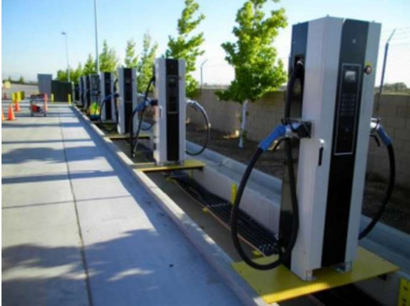
Figure 26: Depot charging cabinets at Antelope Valley 35
