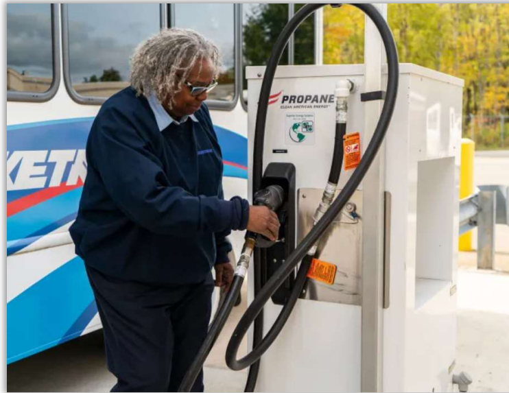
Figure 30: Propane Fueling Infrastructure 45
