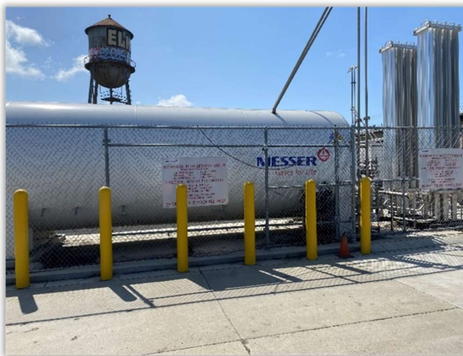
Figure 29: Hydrogen storage infrastructure at AC Transit 42
