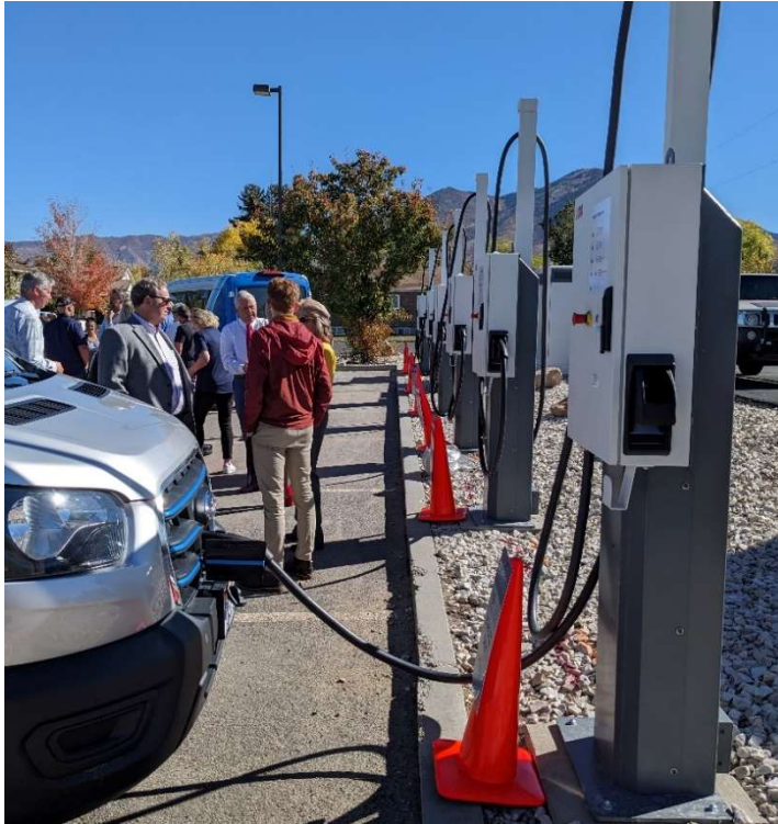
Figure 27: UTA Tooele County On-Demand Fleet Charging
